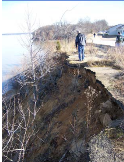
Seth Berry inspects severe erosion immediately adjacent to base buildings at the Phase I project site.
