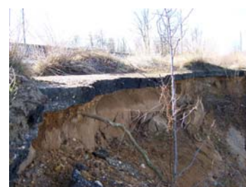
A road undercut by erosion at the
